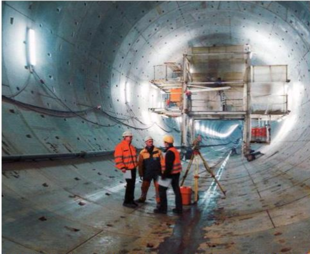
Completed tunnel with linings. From here, 1st stage concrete, rail track, ventilation, electrical and other cables, etc., starts installation.
