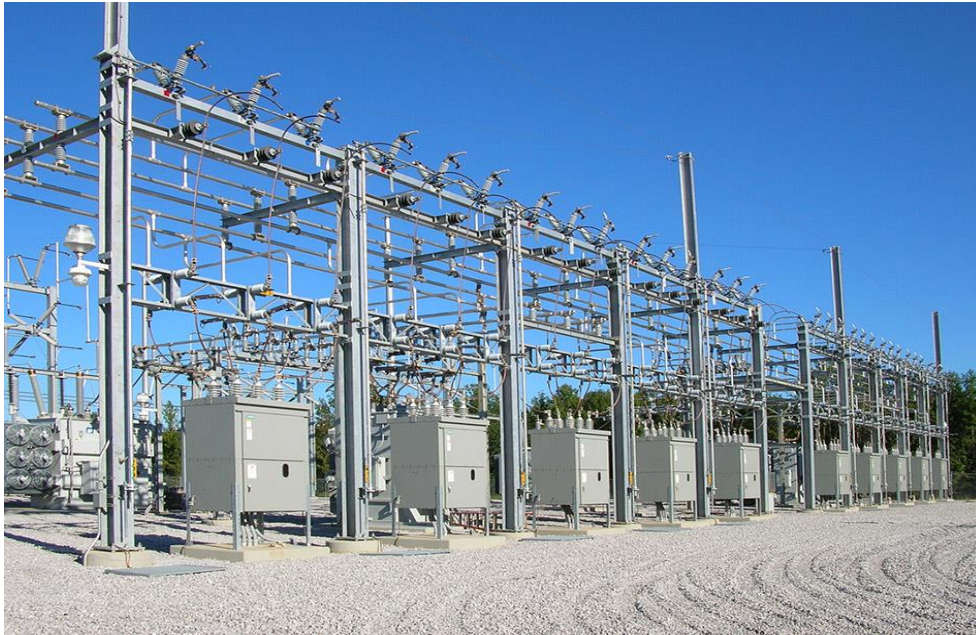
Figure 90. Typical high voltage receiving sub-station
