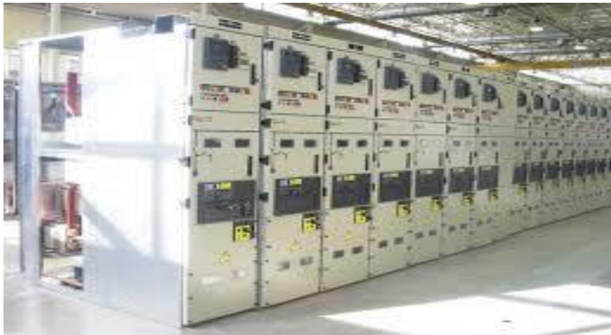
Figure 91. Typical Indoor Auxiliary Sub-station
