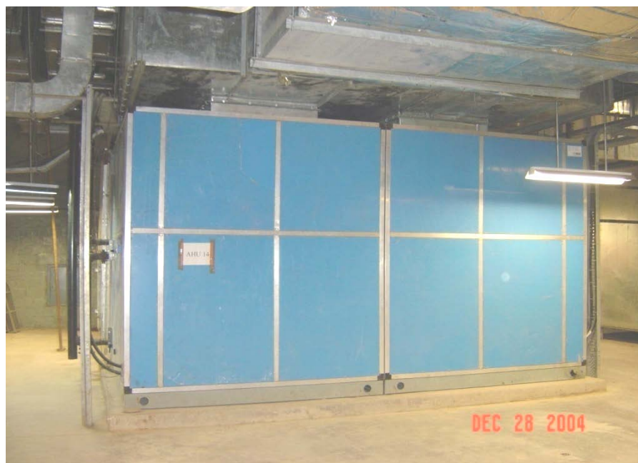
Concourse Air Handling Unit
