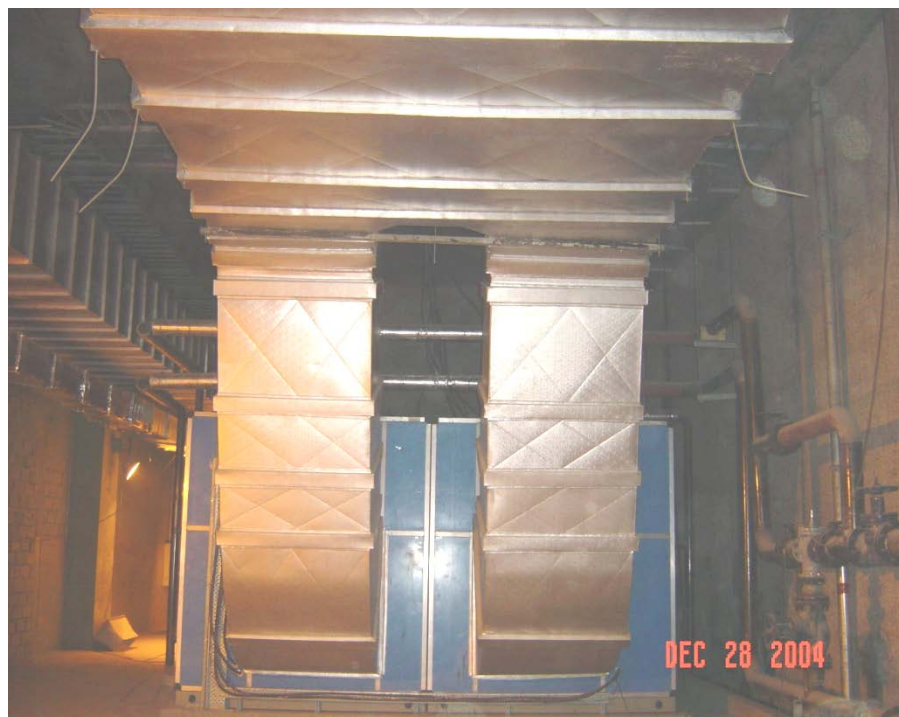
Platform Air Handling Unit
